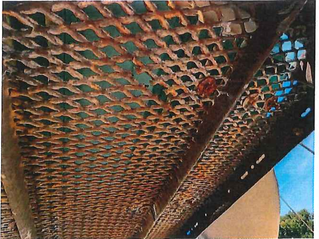
26. CORROSION UNDER DROP SLIDE PLATFORM
