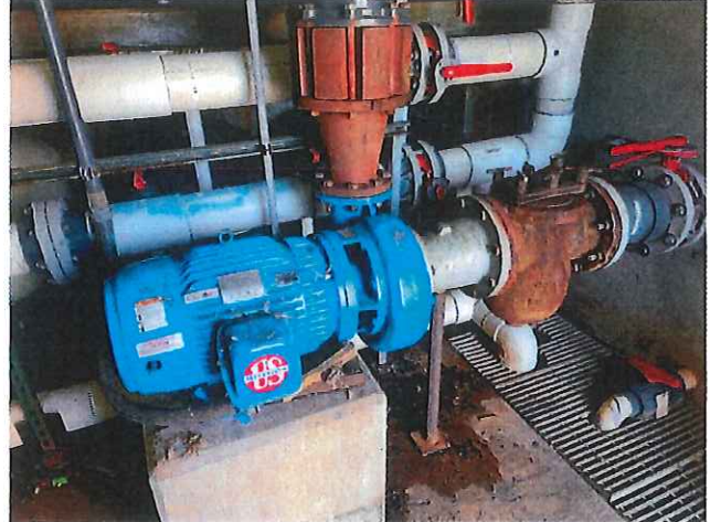
28. CORROSION ON RECIRCULATION PUMP ASSEMBLY
