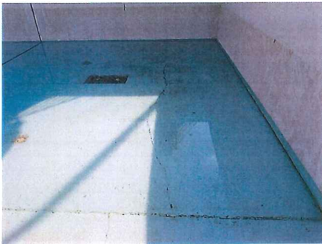
17. CRACK IN DIVING HOPPER
