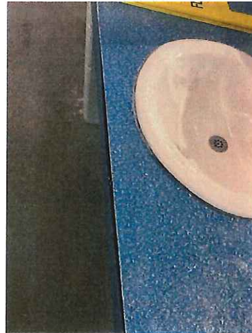
56. DELAMINATING COUNTERTOP AT WOMEN'S LOCKER ROOM
