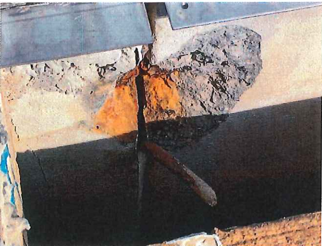
13. BROKEN GUTTER JOINT
