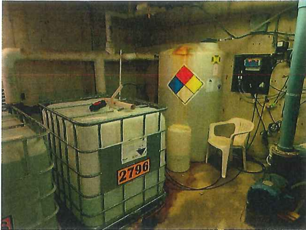
33. CHEMICAL FEED EQUIPMENT
