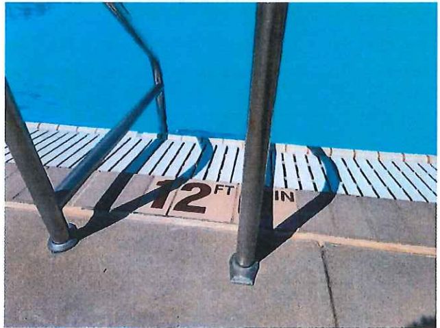
6. CORROSION ON POOL LADDER
