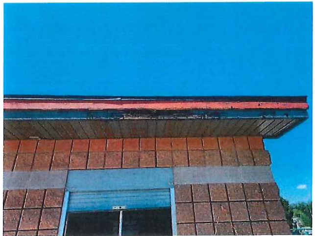
48. WOOD FASCIA BOARD DETERIORATING
