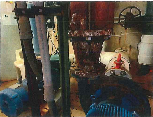
35. HEAVILY CORRODED REDUCER
