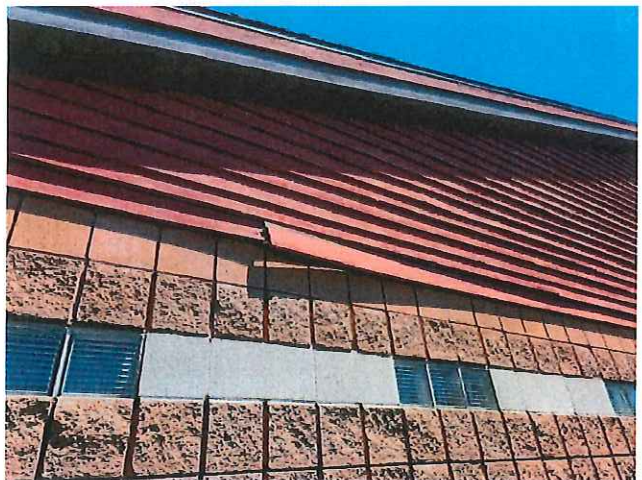
44. WOOD SIDING NOT ATTACHED
