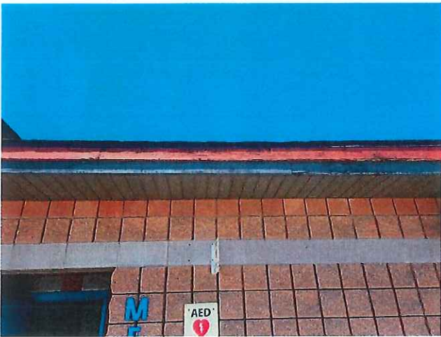
47. WOOD FASCIA BOARD DETERIORATING
