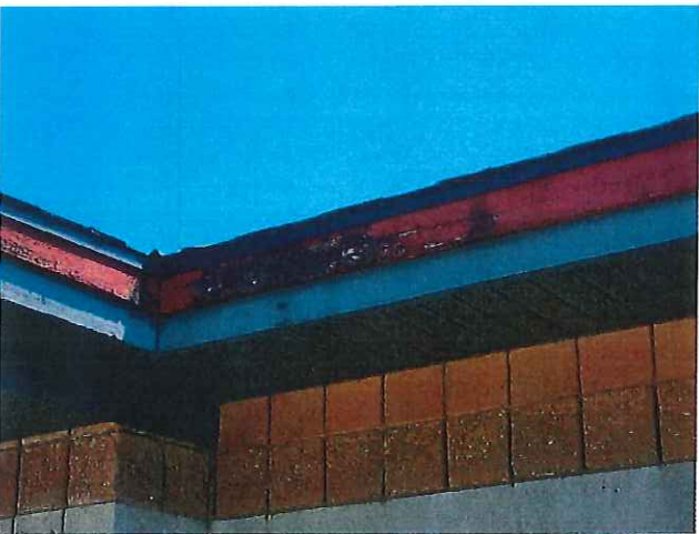
49. WOOD FASCIA BOARD DETERIORATING
