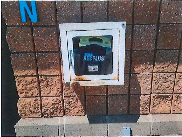
51. CORRODED AED CABINET
