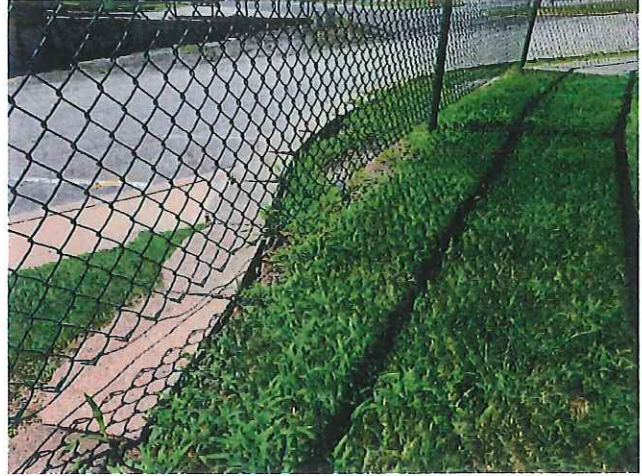
16. GAP UNDER FENCING LARGER THEN 4"
