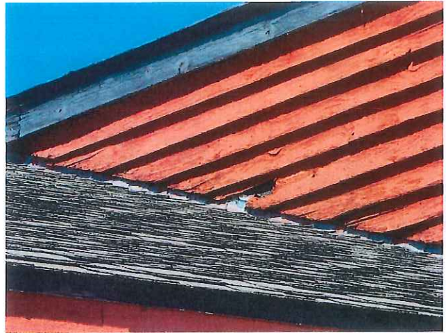
46. WOOD SIDING DETERIORATING
