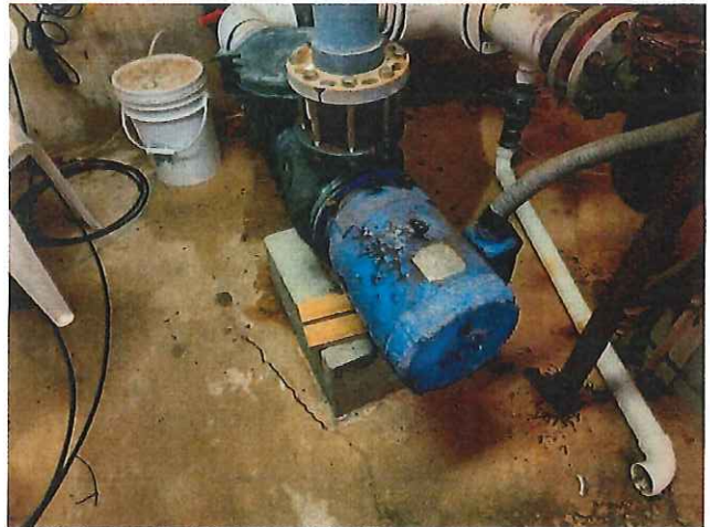
30. CORROSION ON FEATURE PUMP ASSEMBLY
