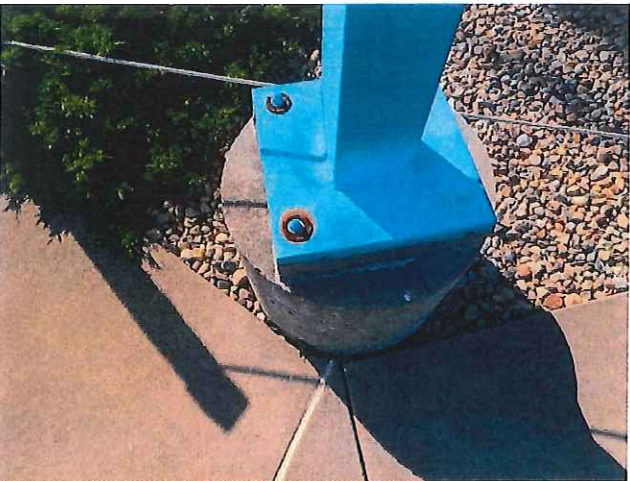
25. EXPOSED FASTENERS OUTSIDE OF BARRIER
