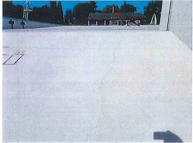
18. CRACK ON TRANSITION PANEL
