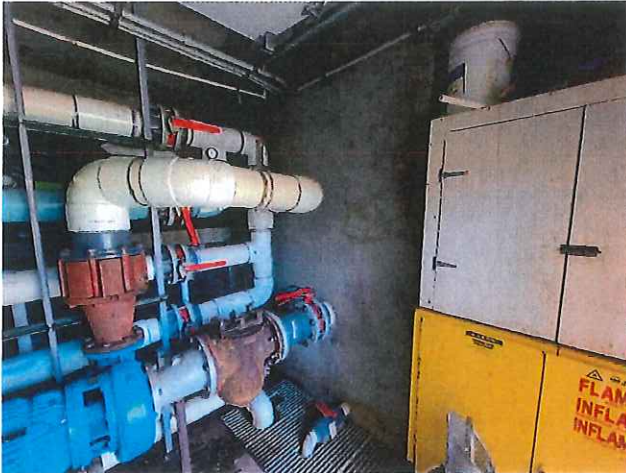
27. SURGE TANK IN MECHANICAL ROOM
