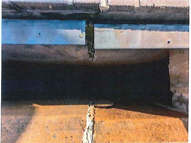
14. BROKEN GUTTER JOINT
