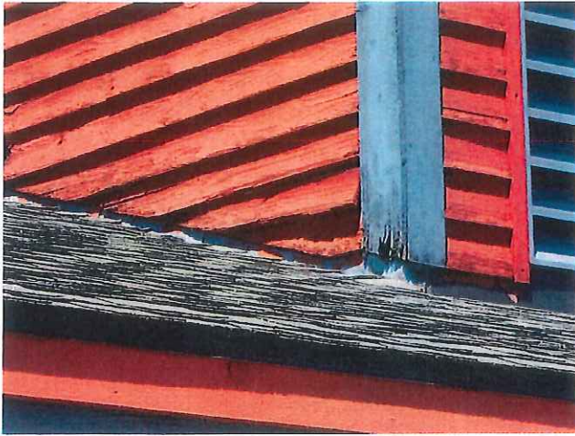
45. WOOD SIDING DETERIORATING
