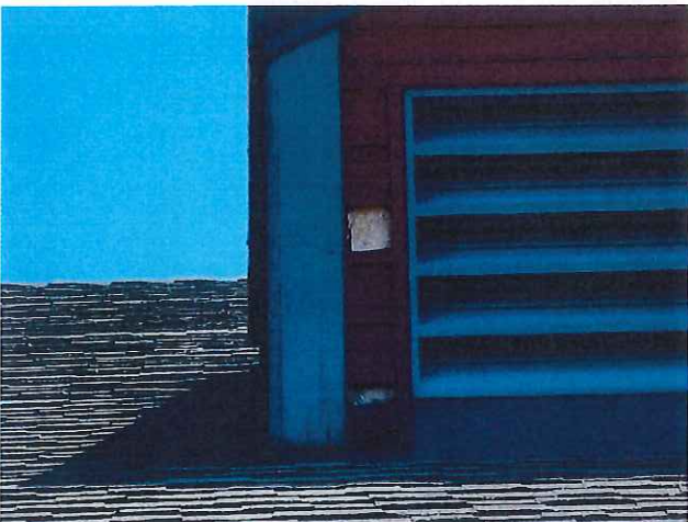
43. MISSING WOOD SIDING
