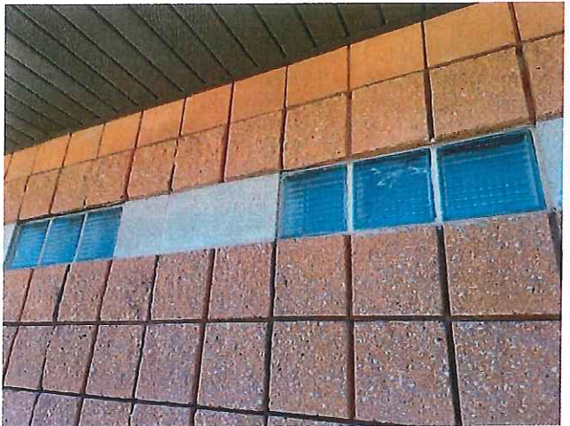
50. BROKEN GLASS BLOCK
