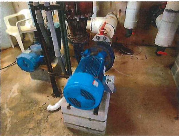
29. CORROSION ON WATERSLIDE PUMP ASSEMBLY
