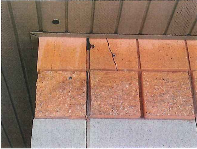
39. CRACKS AND SEPARATION OF CMU
