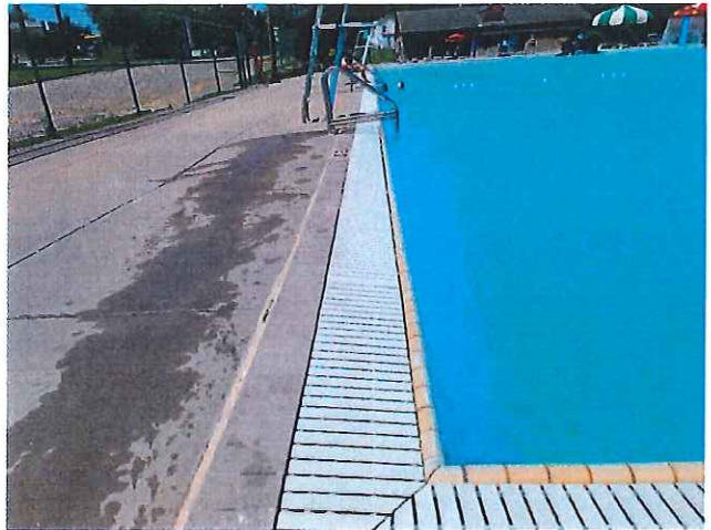
20. NO RIM FLOW OVER GUTTER
