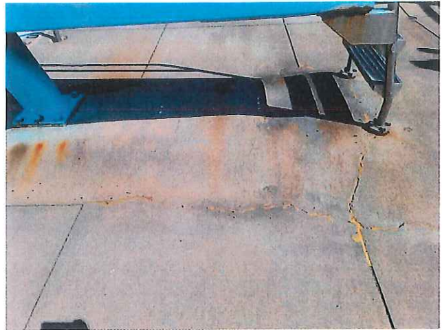
10. CRACKING AROUND DIVING BOARD BASE
