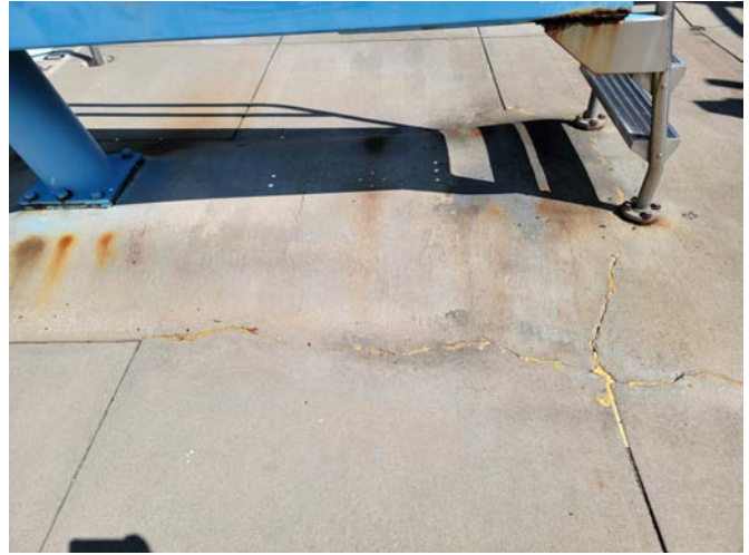
10. CRACKING AROUND DIVING BOARD BASE
