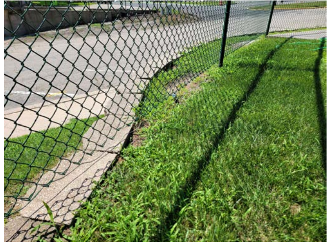
16. GAP UNDER FENCING LARGER THEN 4"
