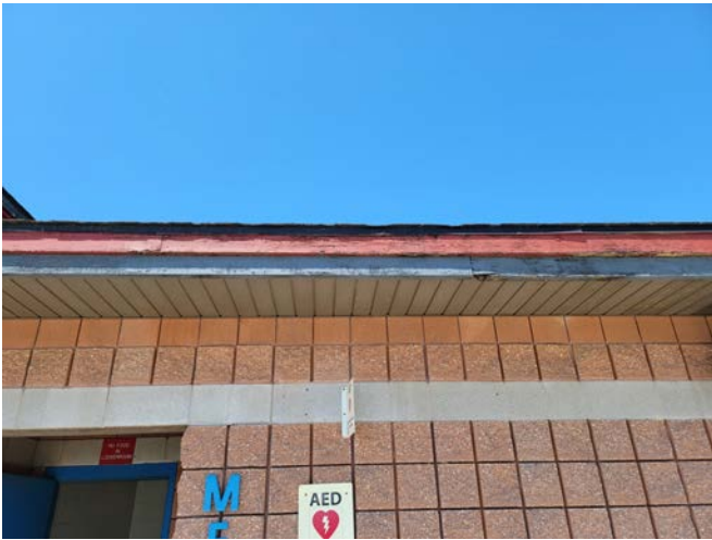
47. WOOD FASCIA BOARD DETERIORATING
