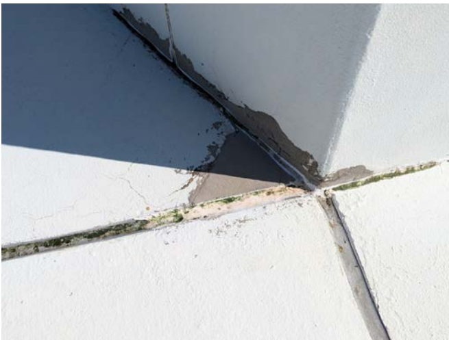
19. FINISH IS COMING OFF THE FLOOR
