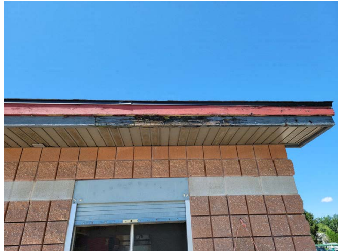
48. WOOD FASCIA BOARD DETERIORATING
