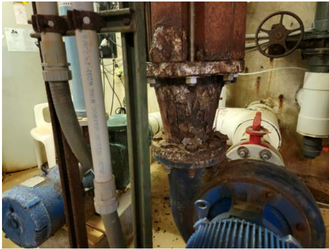
35. HEAVILY CORRODED REDUCER
