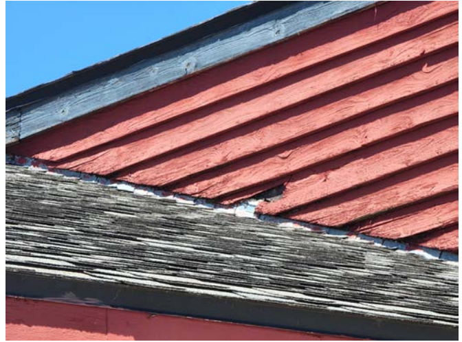
46. WOOD SIDING DETERIORATING
