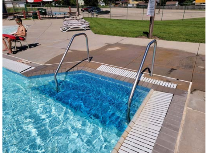
12. WATER OVERFLOWING THE POOL STAIRS
