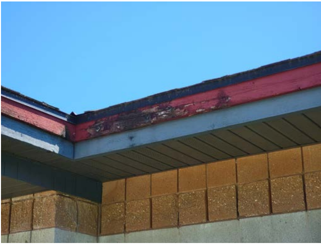
49. WOOD FASCIA BOARD DETERIORATING
