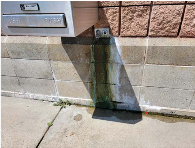
41. MINERAL DEPOSITS AT WATER BIB
