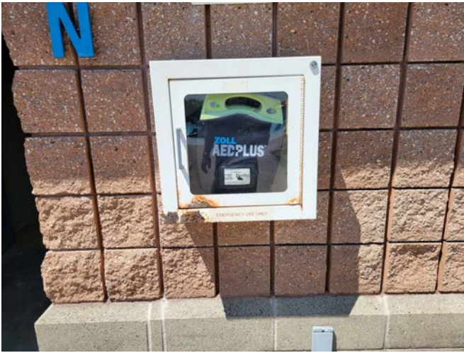
51. CORRODED AED CABINET
