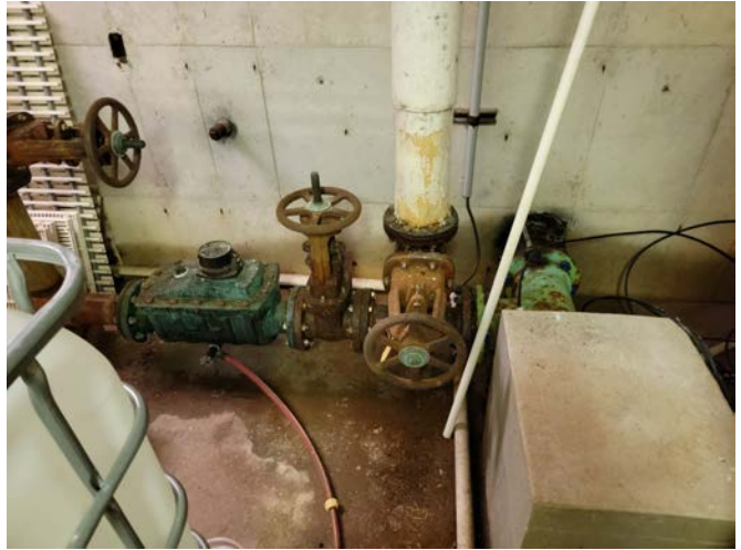
36. CORRODED BATHHOUSE WATER TRAIN ASSEMBLY
