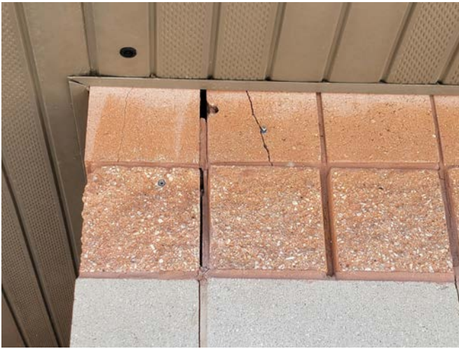
39. CRACKS AND SEPARATION OF CMU
