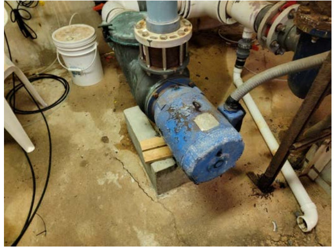
30. CORROSION ON FEATURE PUMP ASSEMBLY
