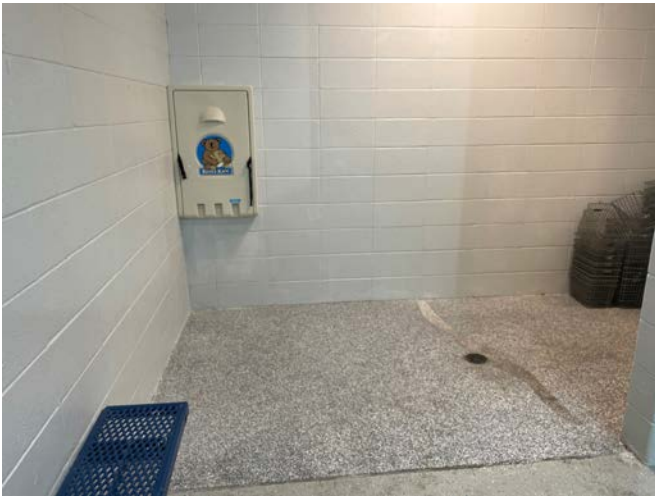
53. CRACK IN FLOOR
