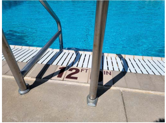
6. CORROSION ON POOL LADDER
