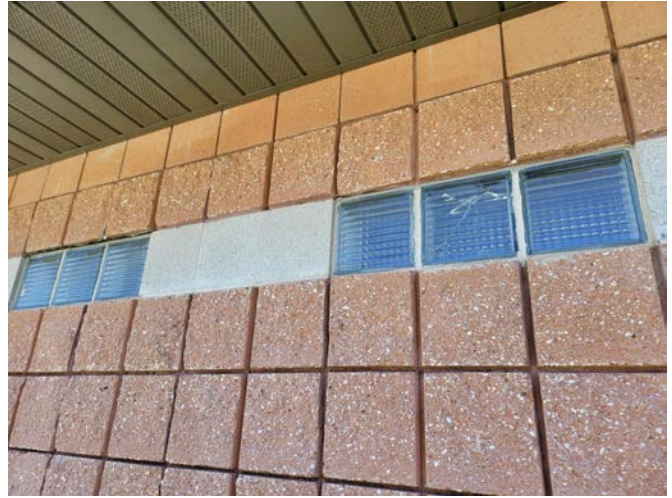
50. BROKEN GLASS BLOCK
