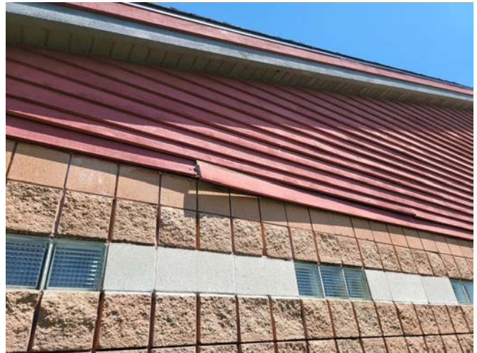
44. WOOD SIDING NOT ATTACHED
