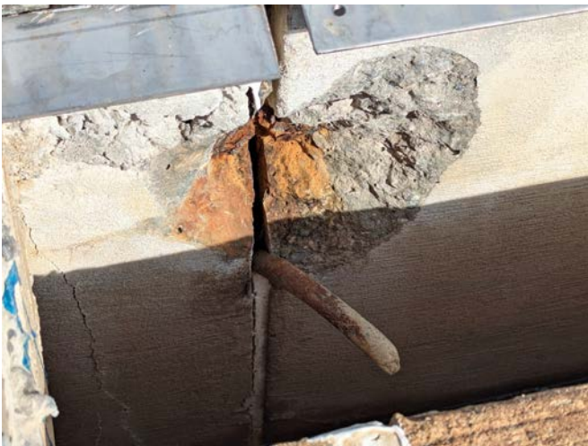
13. BROKEN GUTTER JOINT
