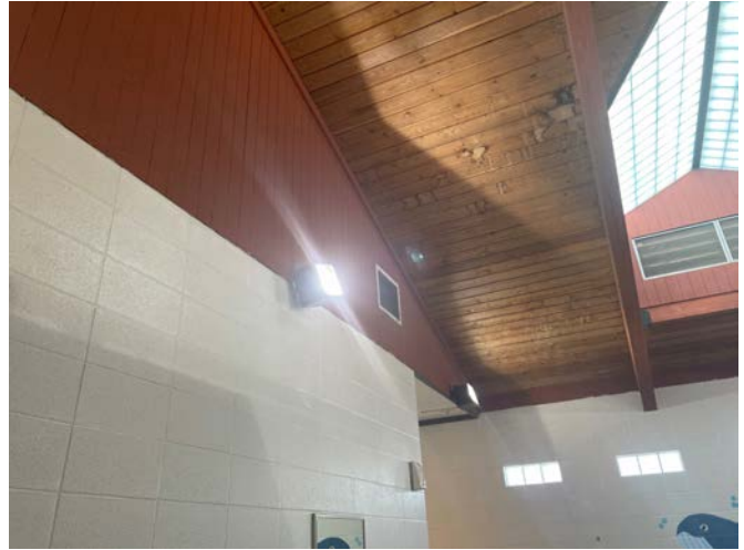
54. DISCOLORATION AROUND SKY LIGHT
