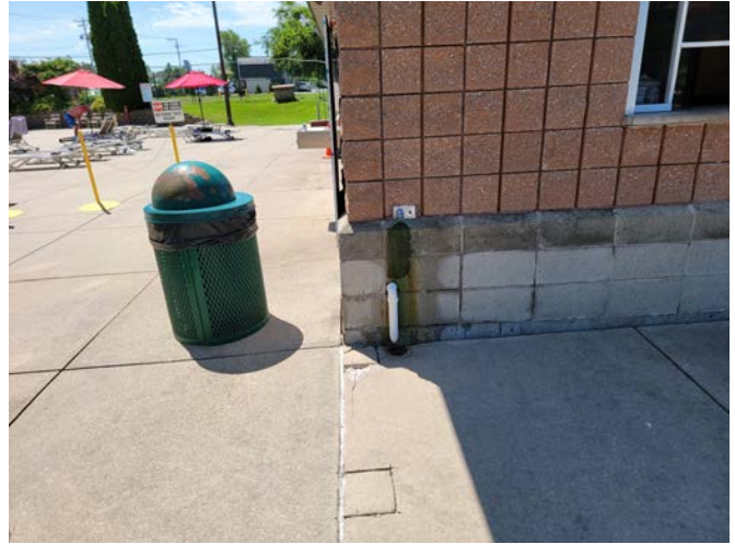
42. MINERAL DEPOSITS AT WATER BIB
