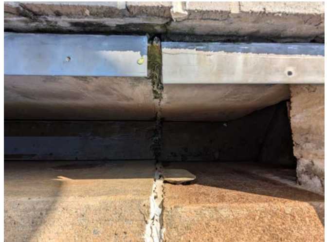
14. BROKEN GUTTER JOINT
