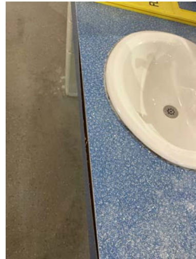
56. DELAMINATING COUNTERTOP AT WOMEN'S LOCKER ROOM
