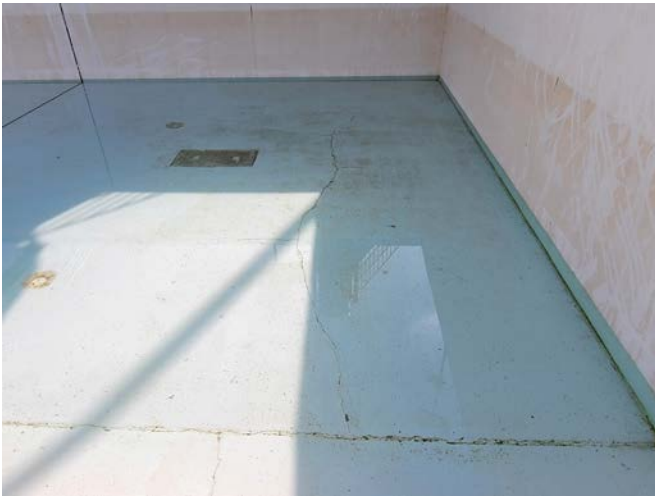
17. CRACK IN DIVING HOPPER
