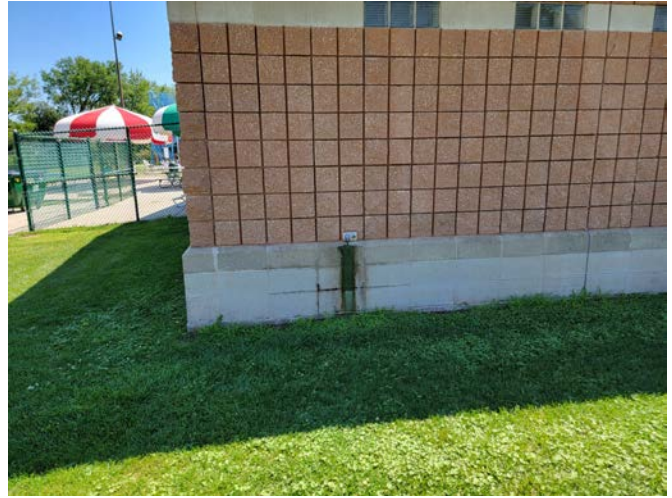
40. MINERAL DEPOSITS AT WATER BIB
