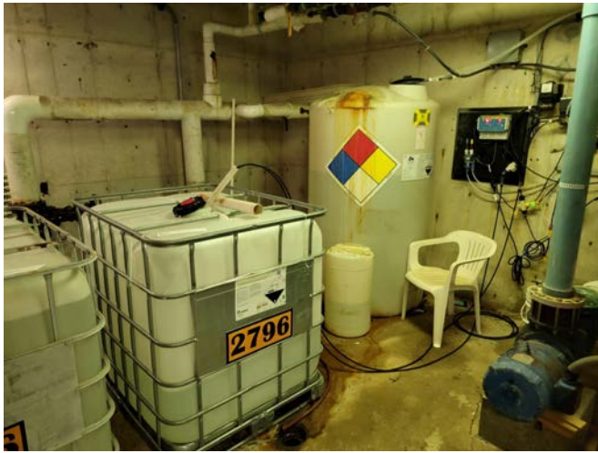
33. CHEMICAL FEED EQUIPMENT
