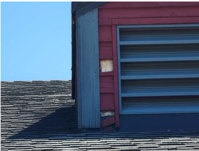
43. MISSING WOOD SIDING
