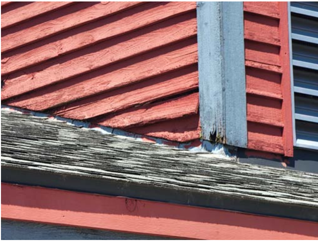
45. WOOD SIDING DETERIORATING
