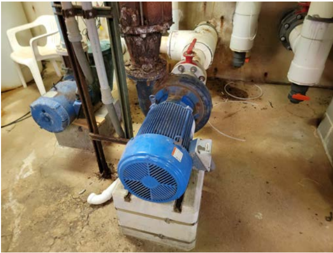
29. CORROSION ON WATERSLIDE PUMP ASSEMBLY
