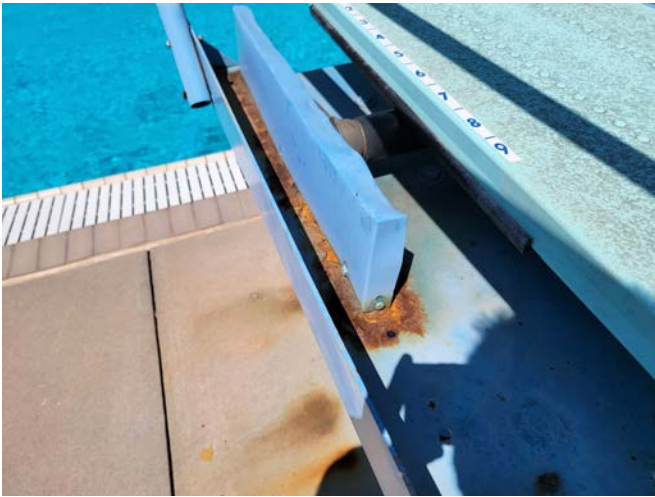
11. CORROSION ON DIVING BOARD ASSEMBLY
