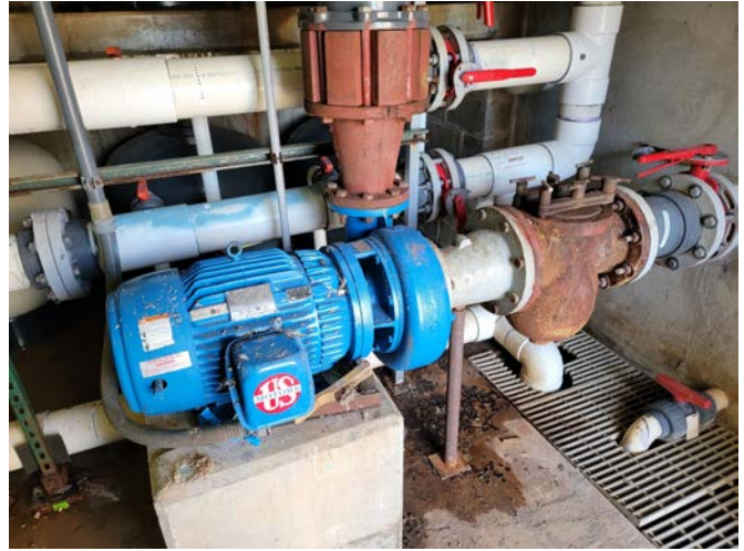
28. CORROSION ON RECIRCULATION PUMP ASSEMBLY
