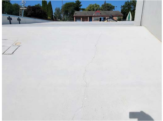
18. CRACK ON TRANSITION PANEL
