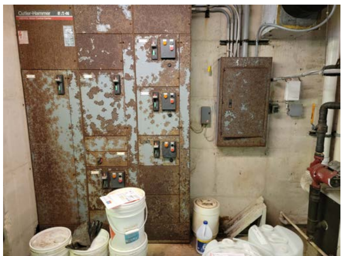
38. CORRODED ELECTRICAL SYSTEM IN MECH ROOM
