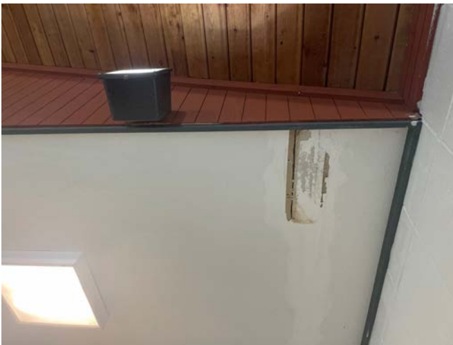
55. DAMAGED CEILING AT MEN'S LOCKER ROOM
