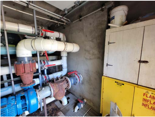
27. SURGE TANK IN MECHANICAL ROOM
